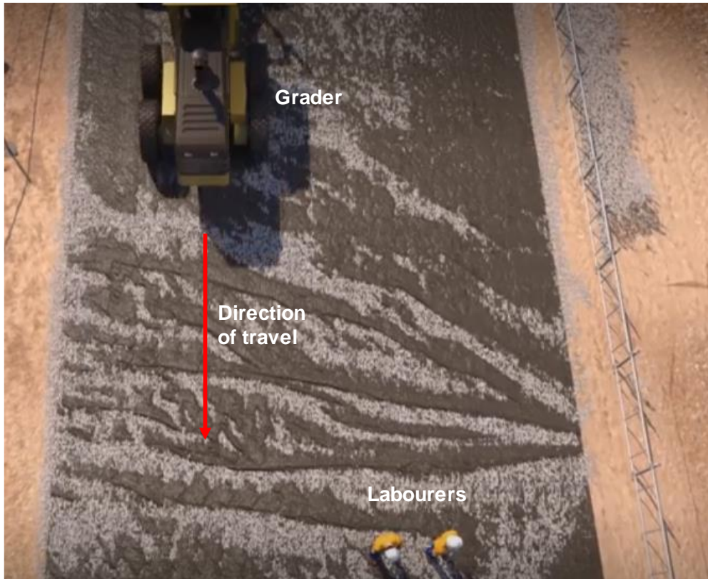
Fig. 2: Aerial view showing direction of travel of the grader and position of the labourers preparing the geotextile fabric on the carriageway.
